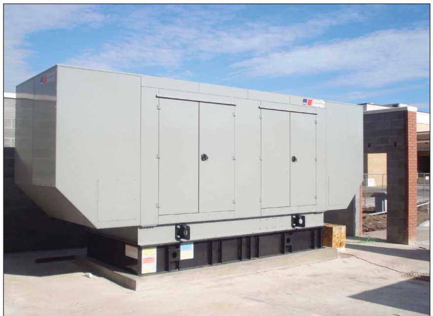
Photo 1. This generator set enclosure includes acoustic barriers and sound insulation enclosures with foam.
