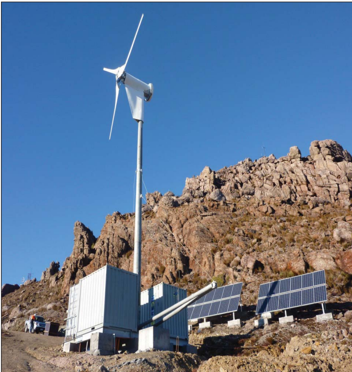
Photo 2. Achieve a lower and predictable opex with outdoor base station units with fans and ventilation, heat-ruggedized base stations and batteries, and mixed renewable energy sources in the form of solar and wind power.
