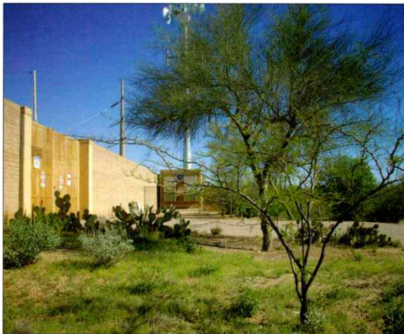
Utility workers access the site through the locked gate seen here in the block wall. In the distance, behind the tree, Crown Castle's tower is visible extending from a position outside the substation perimeter wall, protected by a short wrought-iron fence. The shelter is adjacent to the perimeter wall.
