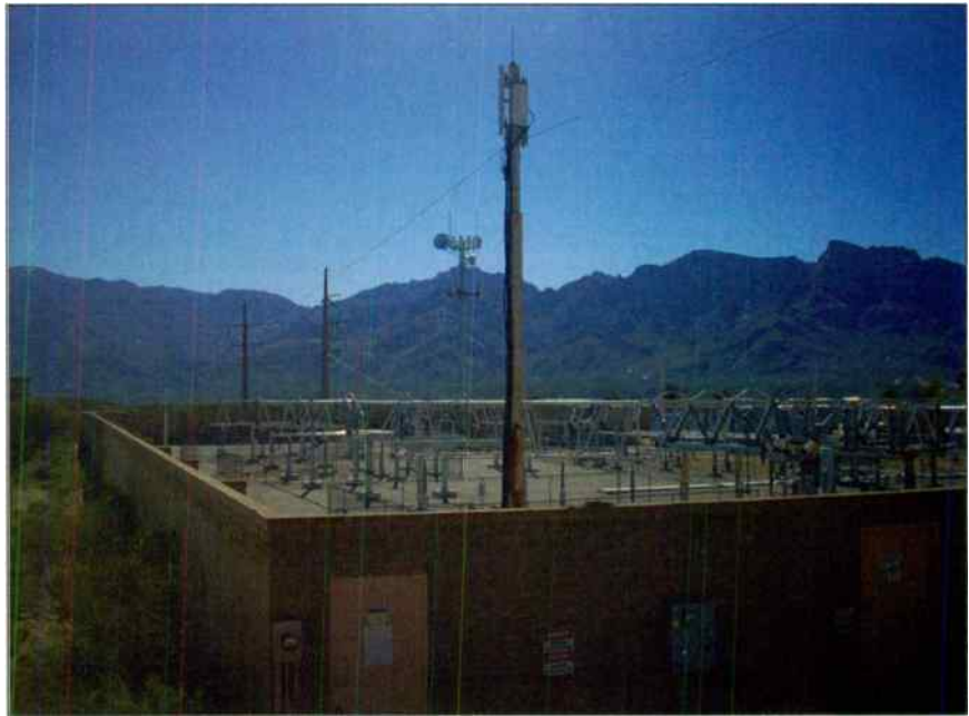
This view shows two of the four towers located on the substation property. One is outside the concrete fence and the other is inside.
