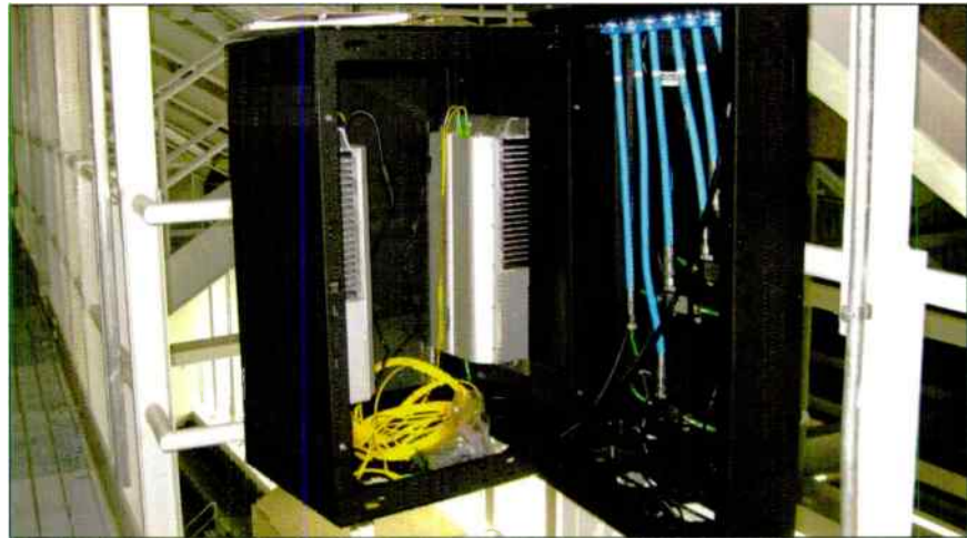
Two intelligent optical network (ION) remote units installed in a box on the catwalk in Cowboys Stadium support the antennas that spread wireless signals throughout the upper concourse. Photo: Andrew Corporation.
