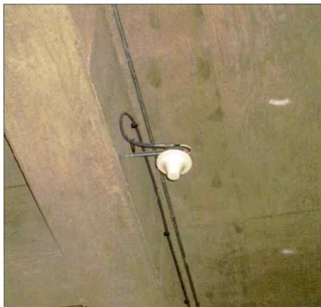
Half-inch coaxial cable feeds a typical indoor DAS antenna mounted in an underground parking garage to deliver wireless services where signals otherwise could be too weak.
