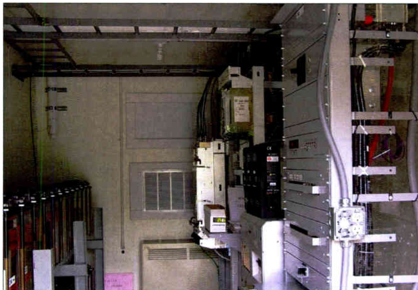
A view inside the cell site shows all the electrical and radio components. At the left is the solar-power battery rack. In the center is a vent and below that is a propane heater. On the right, closest to the far wall, is the Nortel cellular radio. In the second rack on the top is the microwave radio. Black boxes on the third rack are charge controllers. The tall, silver panel in the closest rack contains circuit breakers.
