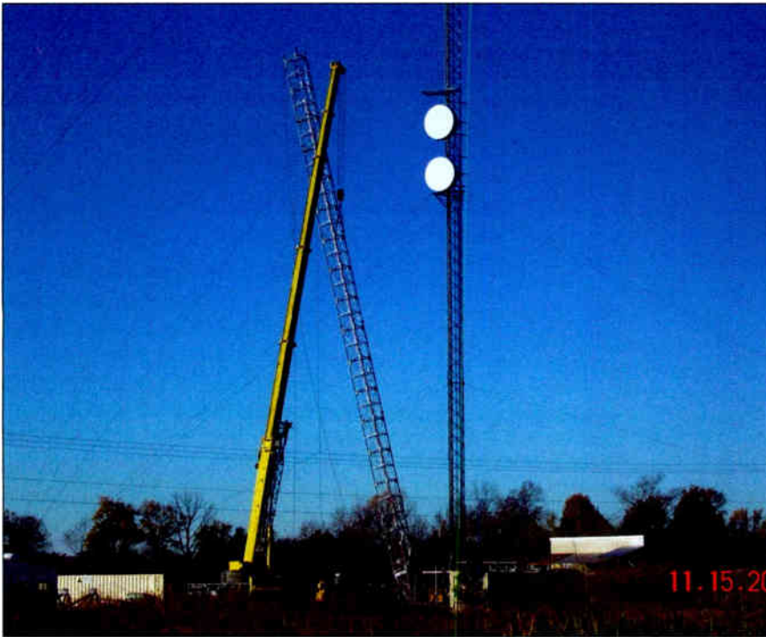
With the use of a crane, the stub was lifted and positioned for placement on the tower base. This picture was taken from afar as a safety precaution.
