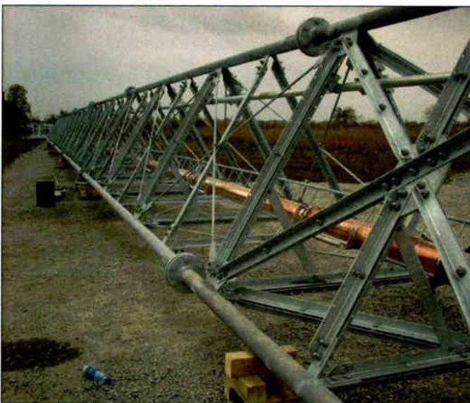
The construction crew finished the first few sections of tower called the stub. A crane erected the stub, and then the crew attached the first guying point.
