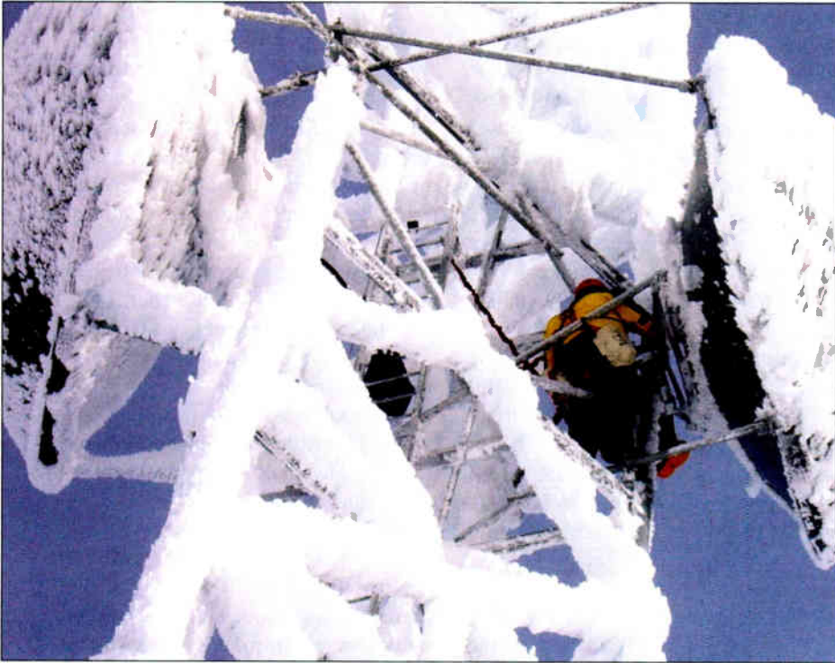
A climber is clearing ice on a telecommunications tower on a mountaintop in Northern California. Ice is a big concern for every aspect of climbing. OSHA addresses requirements for climbing towers during inclement weather. The main concern is that the climber be attached to the tower 100 percent of the time.
