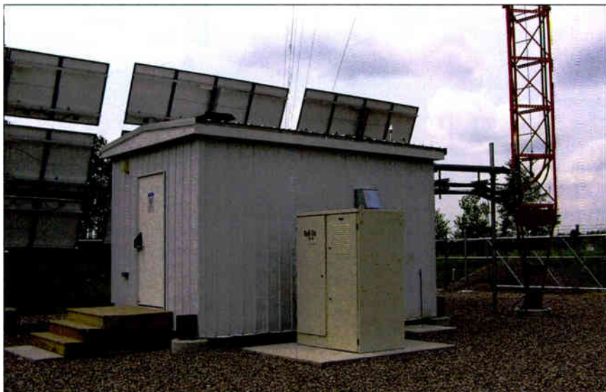
Front and center in the beige enclosure is a ReliOn hydrogen fuel cell that serves as backup to the solar and wind energy producers. The backup gives cell techs 24 hours to reach the site for troubleshooting.
