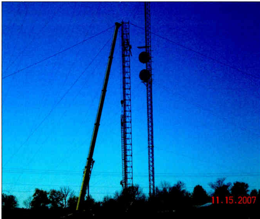
The first guying point was installed by climbers while the gin pole was being hoisted prior to removal of the crane. A close look may reveal climbers working on the gin pole attachment to the tower.
