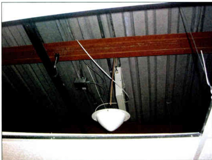
Photo 3. Omnidirectional antennas provide in-building coverage for the Centre's entry hall, dressing rooms, and swimming pool.
