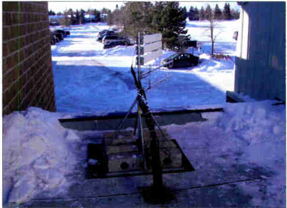
Photo 1. Rooftop masts capture the signal from a distant cell tower for distribution within the Black Gold Centre.
