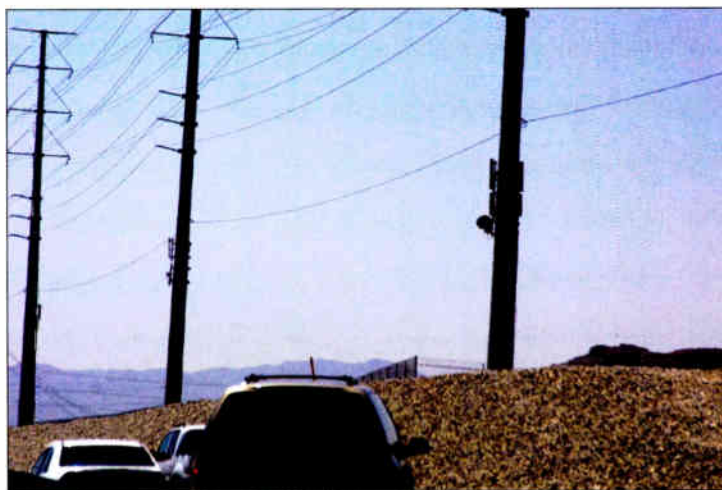
Three transmission poles in a row in Las Vegas, NV, support wireless telecommunications and backhaul antennas.
