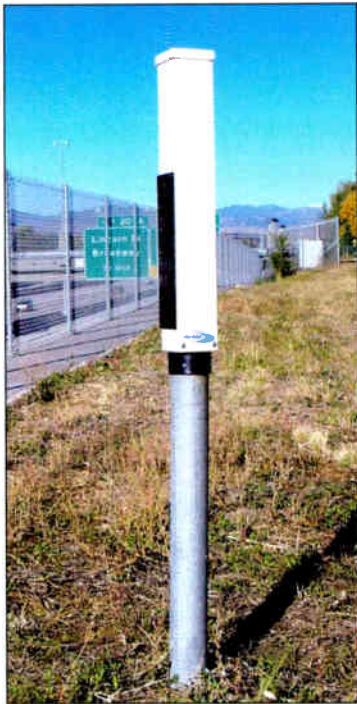
Many operators of buried metal structures are resorting to wide-scale deployment of cathodic protection systems and remote monitoring to ensure their investment in protection and risk aversion stays on line full time.
