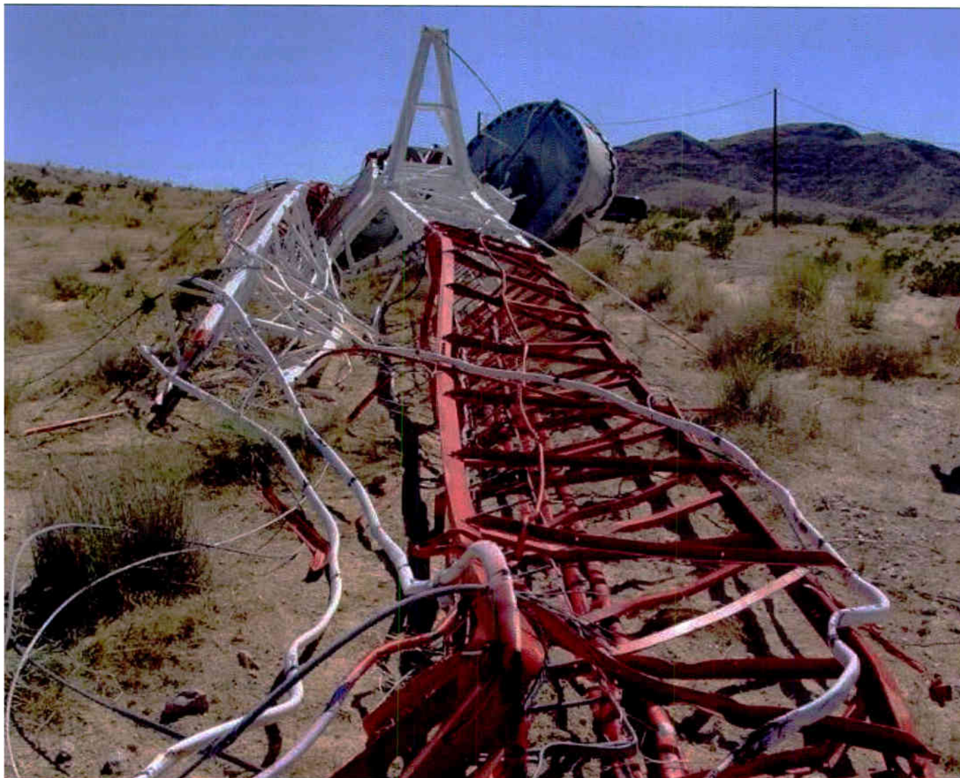
No one wants to come to a tower site to investigate an outage and find this: a mangled tower sprawled across the ground. As towers age, corroded guy anchors pose an ever-increasing risk leading to tower collapse.
