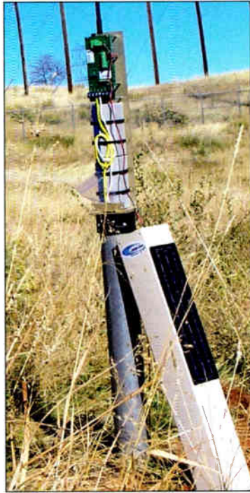
This cathodic protection monitor shows the data radio that monitors the anchor-to-soil ground potential voltage to ensure the sacrificial anode system maintains the tension anchors at the recommended -850 millivolt threshold per NACE standards.
