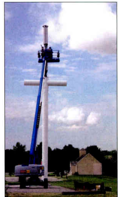
A construction crew places antennas and transmission lines on a cross-shaped tower on church property.
