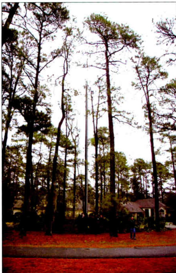
If it were easy to see, it would defeat the purpose. Nestled among the trees and no taller than them is a green-colored treated pole bearing an equipment box near the ground and an antenna on top. The remote access node installation is part of the DAS in Hilton Head Plantation.
