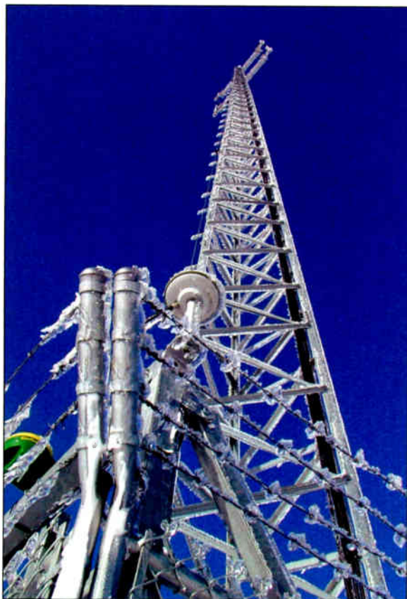
A 100-foot tower at the Casselton, ND, beet-piler site (manufacturer, AN Wireless Tower).
