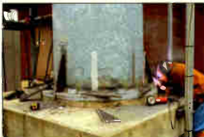
Installation, by a certified welder, of reinforcing base-plate stiffeners to strengthen the base plate.
