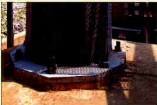
The base plate is shop welded to the monopole shaft in the manufacturer's facility. This weld is the only connection between the monopole shaft and the base plate.
