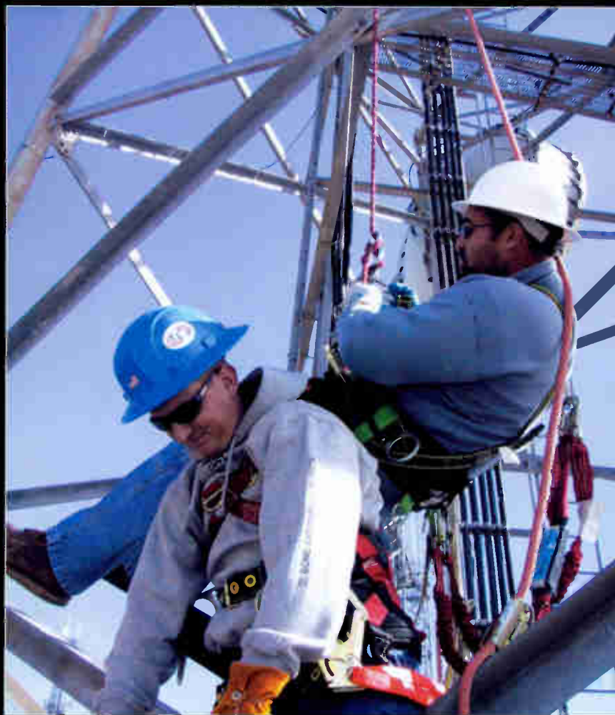
Rescue procedures for extricating a sick or disabled tower climber are an integral part of proper training. Photo courtesy of ComTrain.
