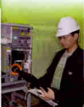
RF Site Solutions
