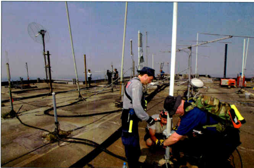
New Orleans, LA, communications specialists from across the country, and FEMA'S Mobile Emergency Response Support (MERS) install antennas on the roof of the 54-story Place St. Charles. Photo by Bob McMilland, FEMA
