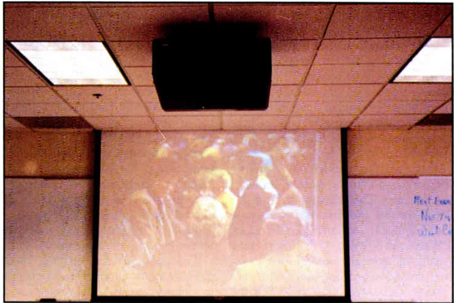
A/V Systems Now's installation of a projection system at Century 21 real estate region V corporate offices in Ontario, California.
