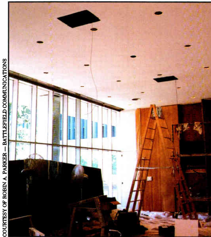
Before and after. These photos show an installation by Battlefield. At left are the rough-in of backboxes. At right, after masking, before paint.
