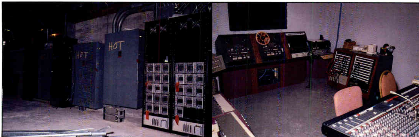
Light dimmers for the church are able to be addressed independently through a Strand system.
