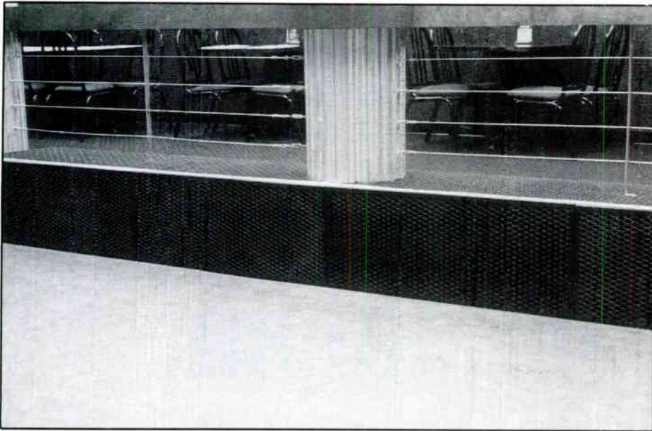
Clair Brothers installed four of the company's own 18-inch ported subwoofers in the City Lights installation.
