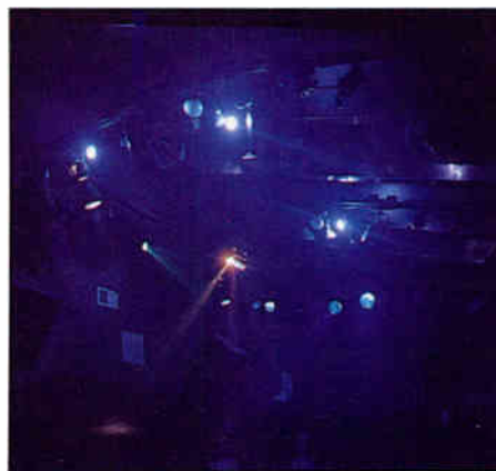
A recent Clair Brothers installation, City Lights Nightclub, contains C.B.A. R2-T 2-way loudspeakers.
