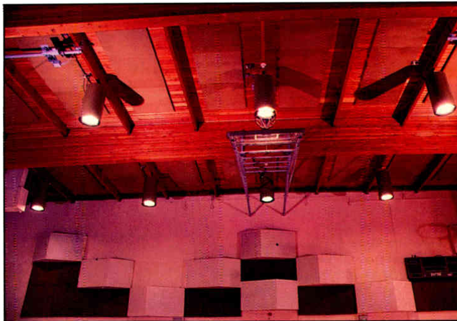
Acoustical absorber/diffusers are mixed with acoustical foam on walls. Note the acoustical foam on the ceiling.
