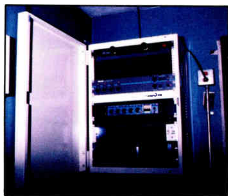
Equipment rack, with a remote power control system permitting unattended single switch operation.
