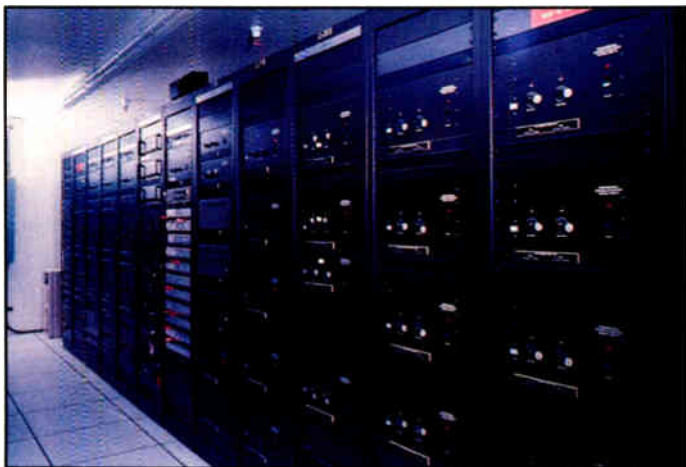
A portion of the music/page power amplifiers used to power speakers throughout the Mirage facility.
