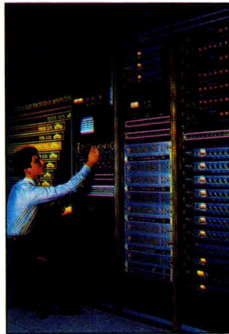
Philip Morris Equipment Room.
