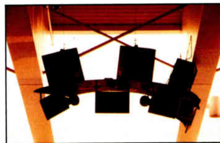
In this front view of the array, it can be seen that the completed array is aimed and positioned as depicted on the drawings.
