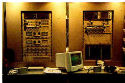
ROH/Metro-Audio control systems.
