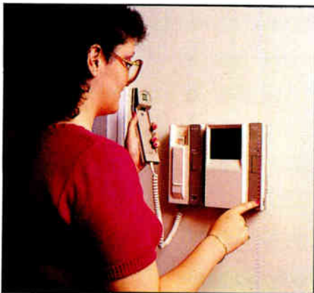
Apartment unit with door release.
