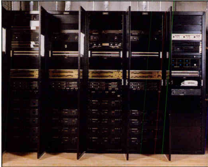
Alumni Arena Equipment Racks
