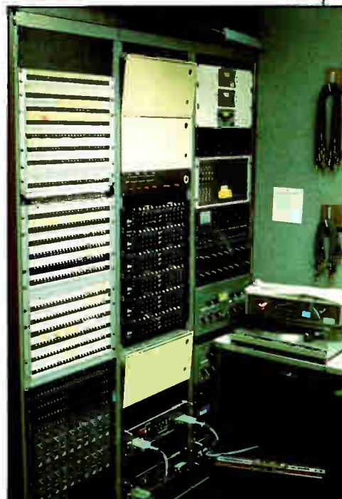
(Top) control room view of stage; (bottom) control room racks with Cetec Ivis and Meyer Sound equipment; (left) view of audience from stage.
