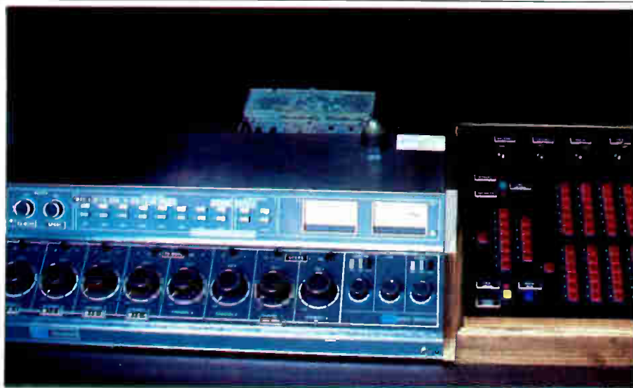
City Council Chamber console and mimic panel.
