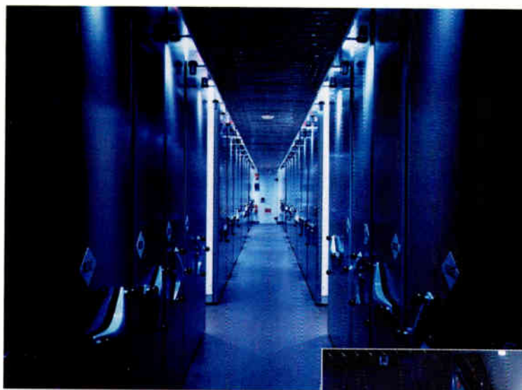
Access to the five main vault rooms, which are filled with high-density shelving units.
