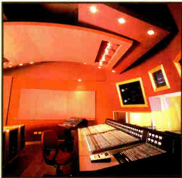
Circo Beat’s control room, with SSL 4056 console and Argentina’s first Genelec 1039 monitors
