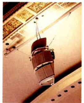
Carnegie Hall A coherent array of UPA-1A loudspeakers, supplemented by MSL-3s and 650-R2 subwoofers (not pictured), is permanently installed for live performance reinforcement.
