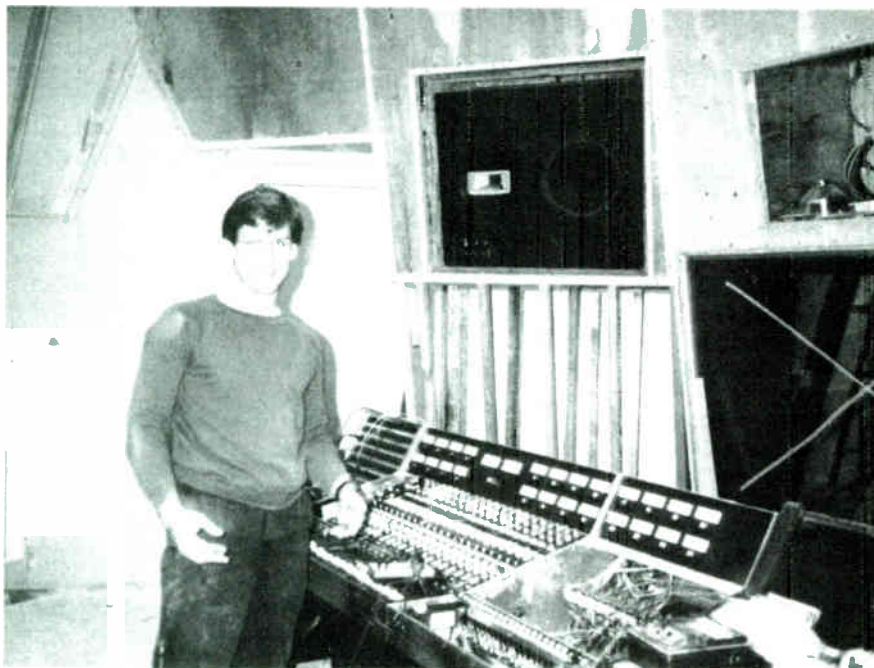
Arley Seeger, Platinum Island's chief of maintenance, installs the modified API console in the unfinished Platinum West control room.
