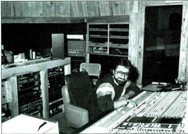
Lakeside Associates of Irvine, CA, designed and built Chartmaker, the private studio of super-producer David Foster in just 11 weeks. It has a comprehensive MIDI interface system, an SSL 4000E console previously owned by the Record Plant, Studer recorders and extensive outboard and video gear. The main monitors are 3-way JBL cabinets designed by Lakeside. Shown here is Humberto Gatica at the console.
