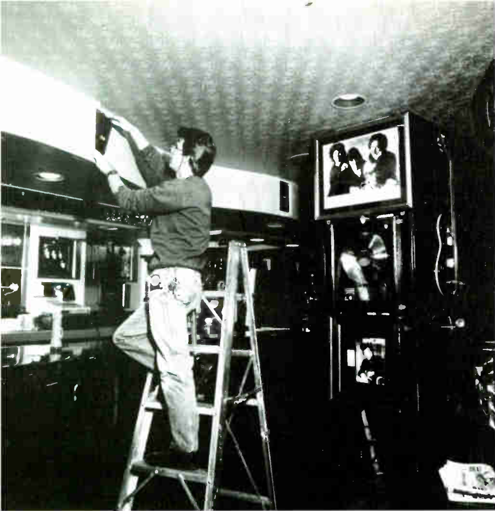
Technician installs one of the 52 Ramsa WS-A 10K speakers used throughout the Hard Rock Cafe into the soffit over the bar.
