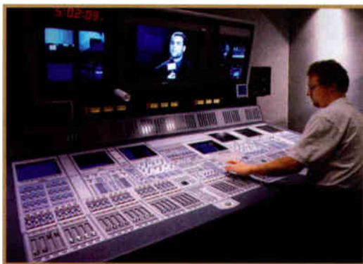
The Sony Oxford console at Staples Center, integrated by A. F. Associates
