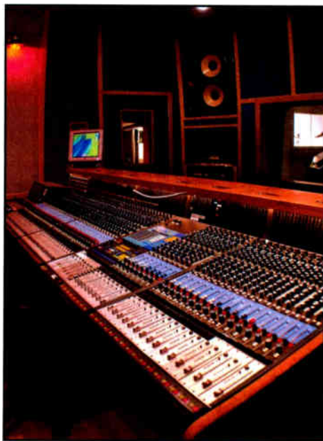
The Headway Music Complex in Westminster, Calif., recently upgraded its Studio 2 with the installation of a 64-input, GML-automated Neve console.
