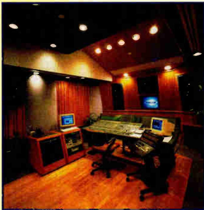
A custom ATC Loudspeakers installation at Sony Music Studios, New York.
