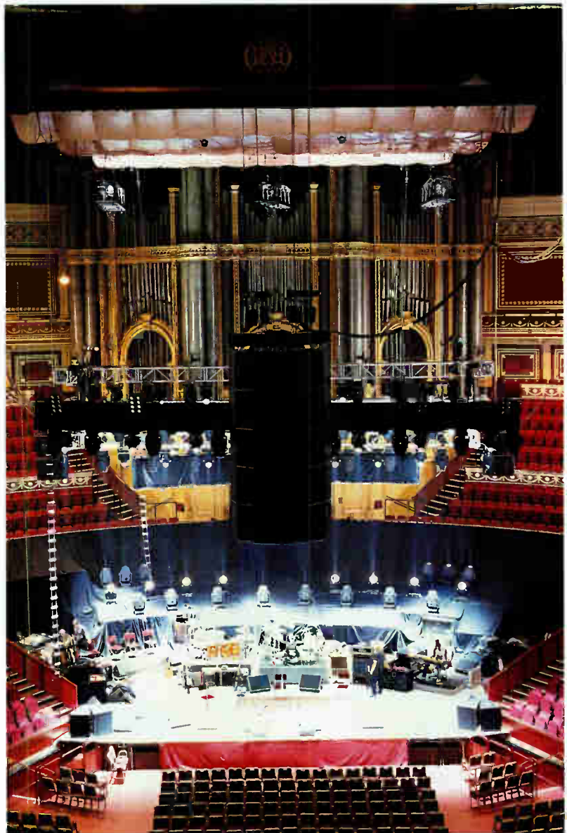
The EAW KF900 system hung as a center cluster. Front section of the audience is covered with ground stacked EAW KF750s.
