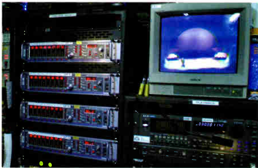
A rack of Aphex Model 1788 remote-controlled mic pre-amps, positioned backstage for Seussical .
