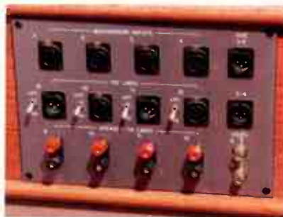
Patch panels located throughout The Cave allow a variety of signals — mic, line, instrument, video, and even speaker level — to be routed anywhere else.
