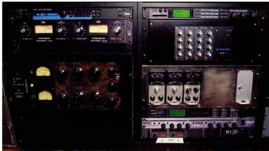
The Bacon Brothers make use of an array of vintage and not-so-vintage gear. On the left side of this rack, there's a Lexicon PCM 70, two UREI LA-3A, and a Fairchild 670. On the right, a TC Electronic Fireworx, an API 550B lunch box with four modules, a Pye Limiter, and a TC Electronic Finalizer, Aphex Compellor, and John Hardy two-channel M1 mic preamp.
