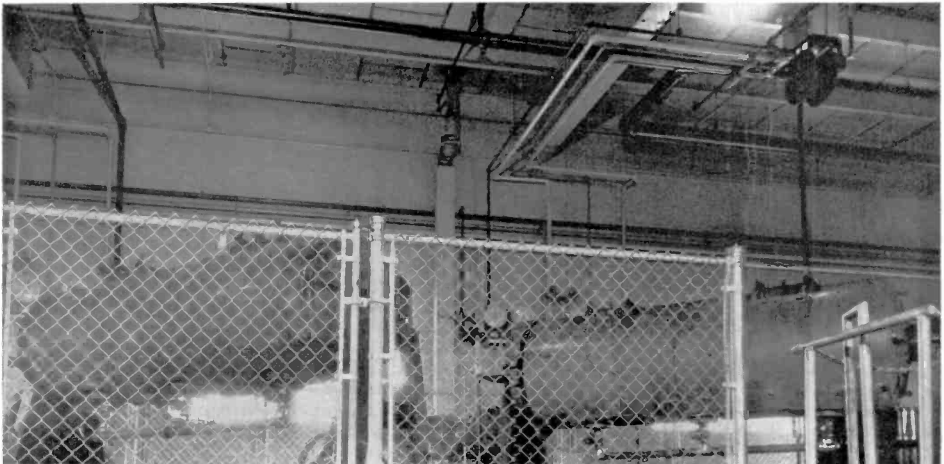
Last step before coating is the milling of the oxide and binder ingredients to produce a homogenous mass without lumps. These ball mills are installed in the new plant of the Reeves Soundcraft Company in Danbury, Connecticut. Like the previous steps in the manufacture of tape, this milling is also a rather critical process.
