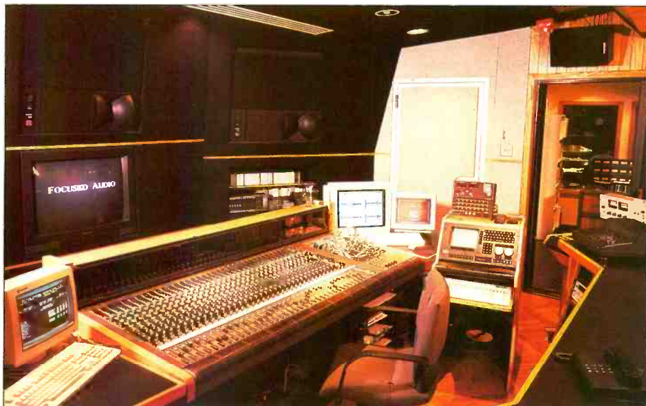
The facility design for Focused Audio, San Francisco, called for four separate mix-to-picture control rooms and a companion audio-video machine room squeezed into just 5,600ft 2 of floor space
