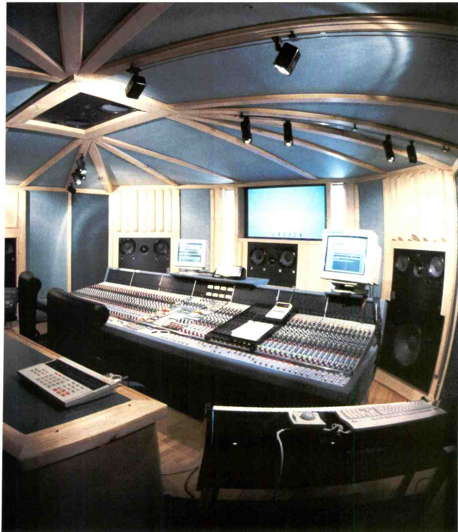
Touchdown Studio 2 showing equipment and monitor installation
