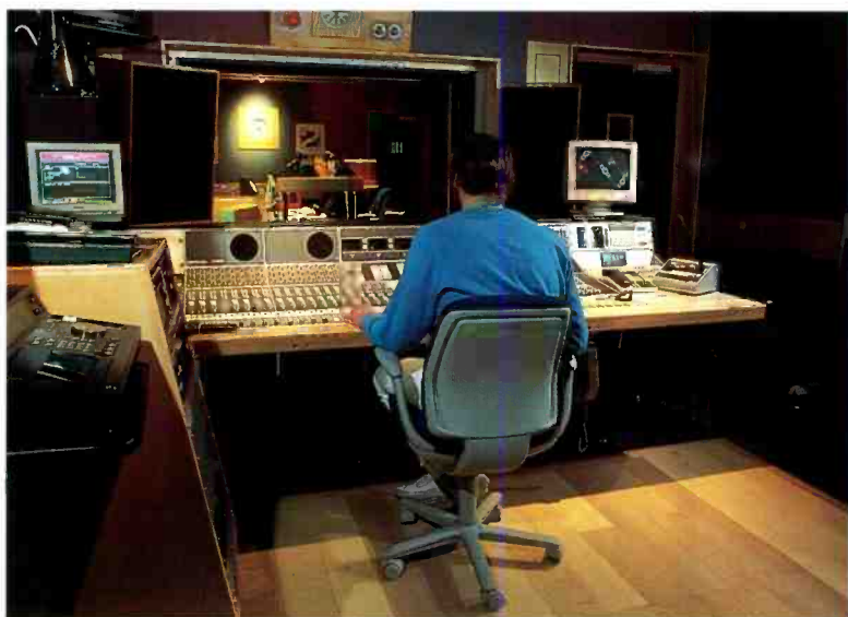
◀ BBC Radio 2 Presenter John Dunn, on-air with the latest of four SL 5000 M Series consoles to be installed in Broadcasting House, London
