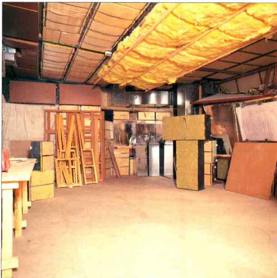
Speaker enclosures are now in place in the main hall Control Room for the hybrid Air-Andy Munro monitors
