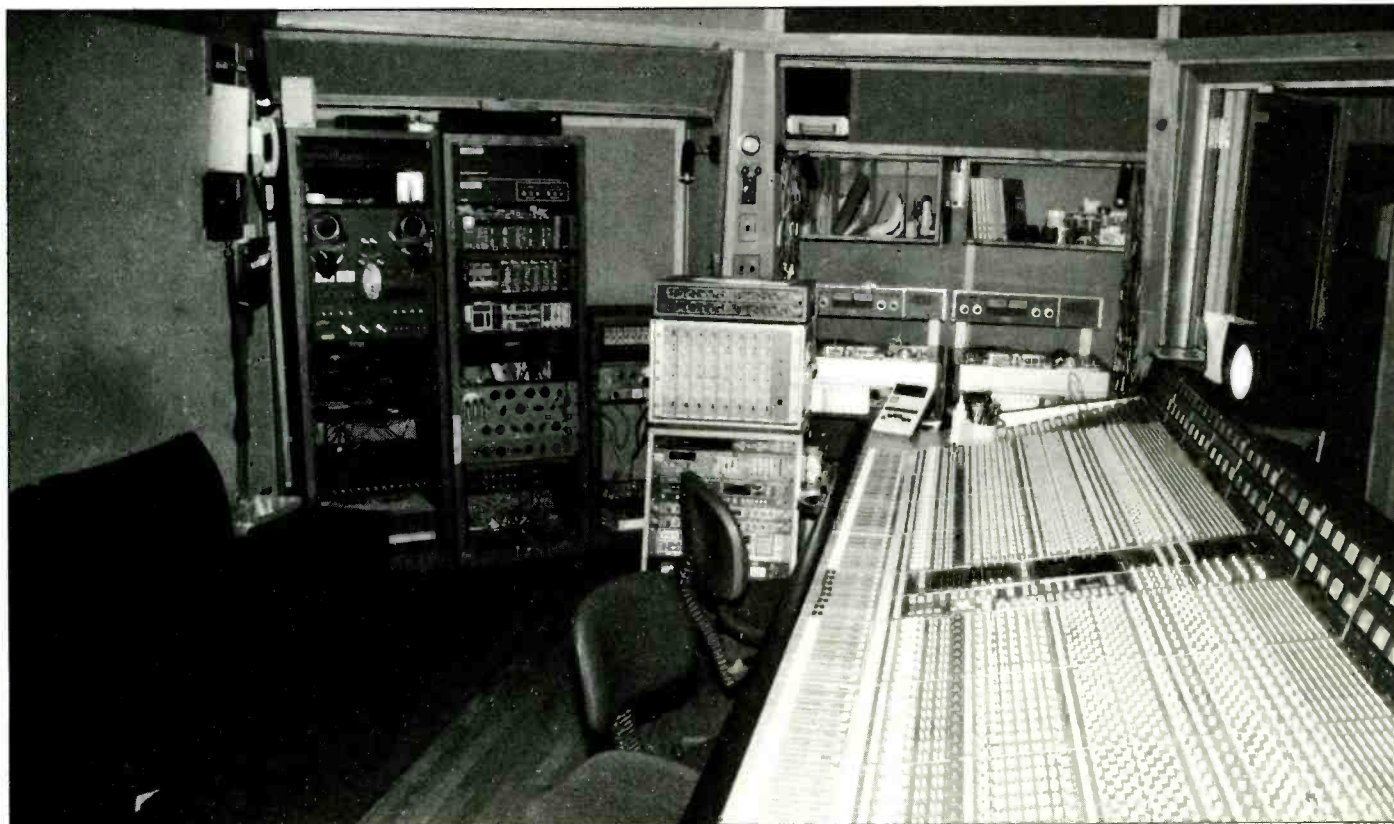
Control Room B
