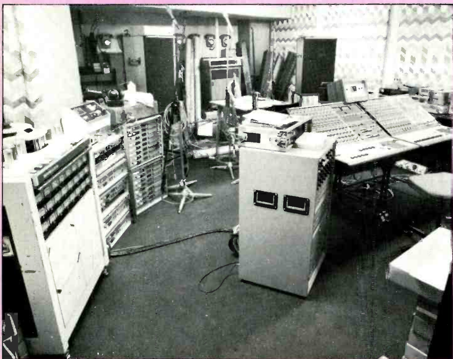
Control room for TRU
