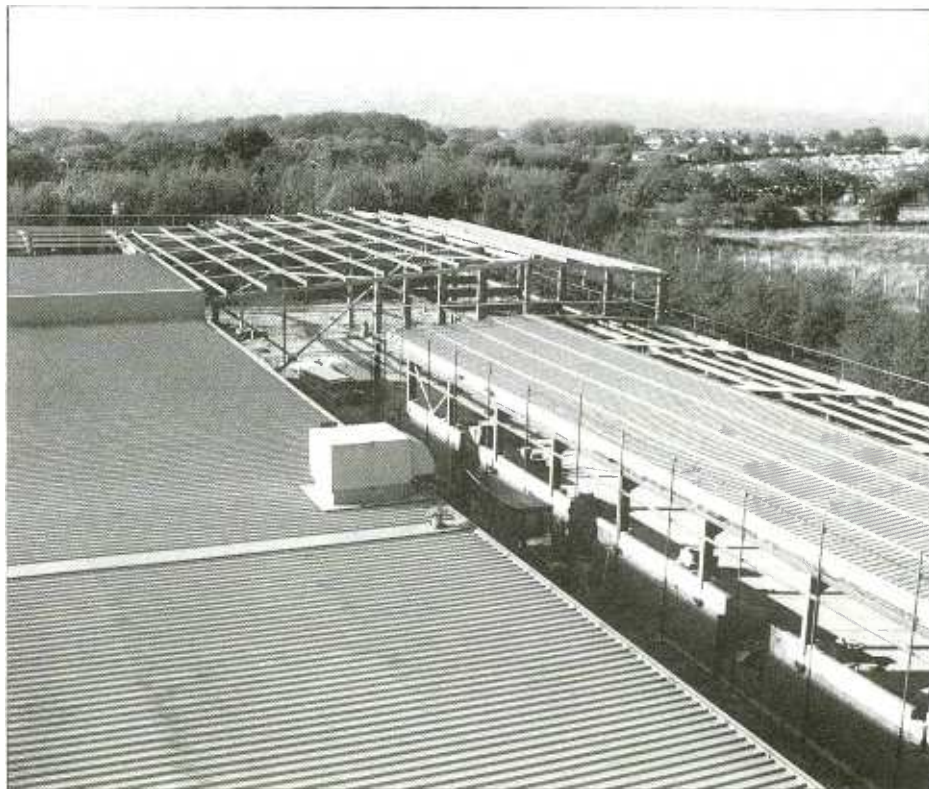
The 22,000 square foot extension on schedule for late summer to accommodate the Calrec Manufacturing Section.
