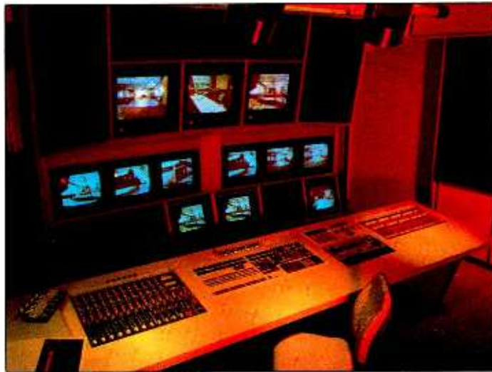
Video control room
