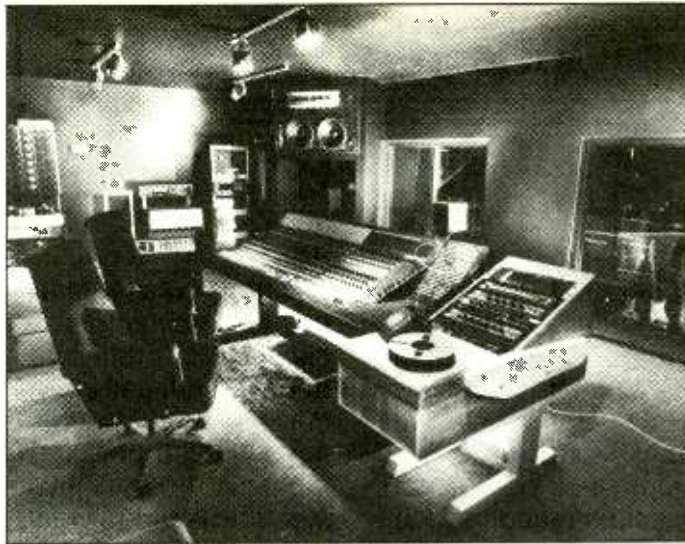
Control room of Regal Sound, Hitchin, a recent project undertaken by Turnkey.
