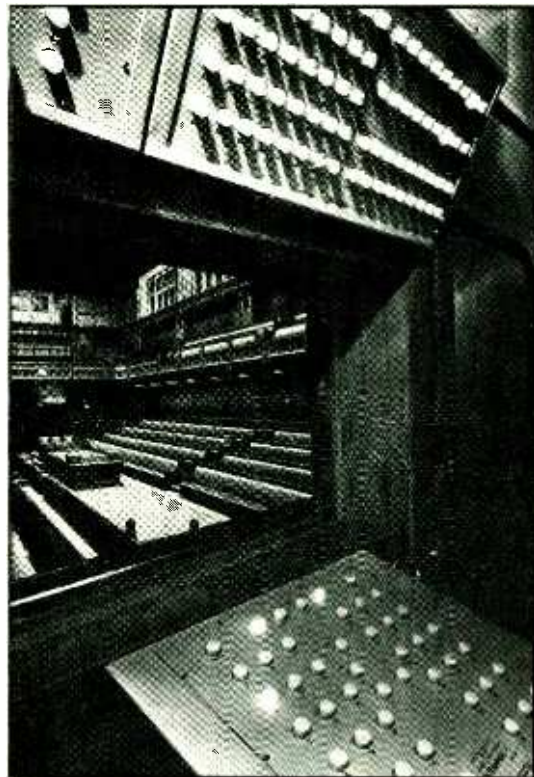
Right: Control room at Westminster
