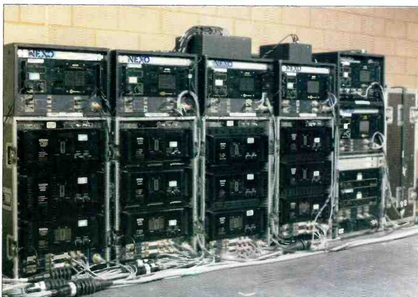
All of the signal sources were routed first to the main racks and then distributed from there to the others via multicores.
