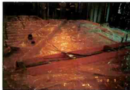
The preparation of NBC's Edit 7 floating isolated floor system, with technical wiring interconnect troughs for the concrete pour.
