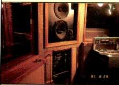
At Blue Jay Recording, the monitor speakers were originally mounted with the power amplifiers directly underneath, causing imaging problems from convected heat. This problem was solved by placing the amplifiers in the central machine room.
