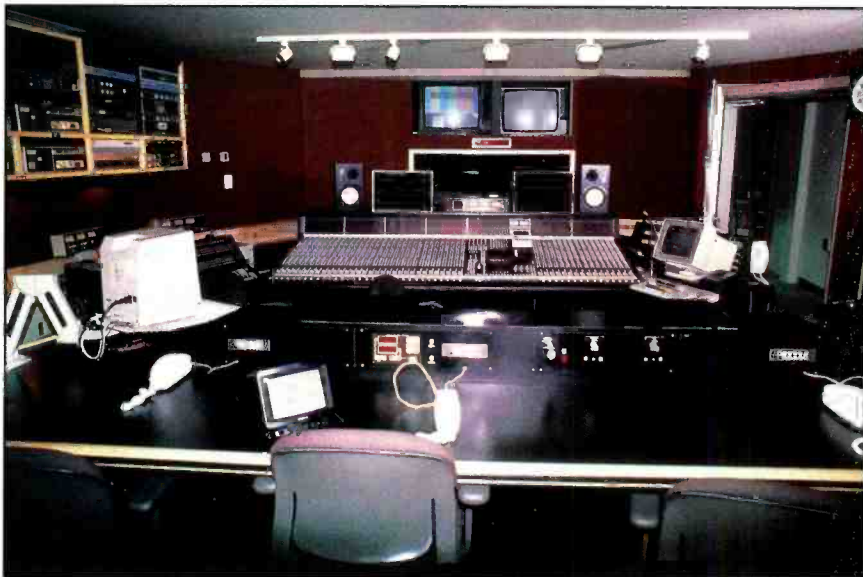
The completed Edit 7 control room.
