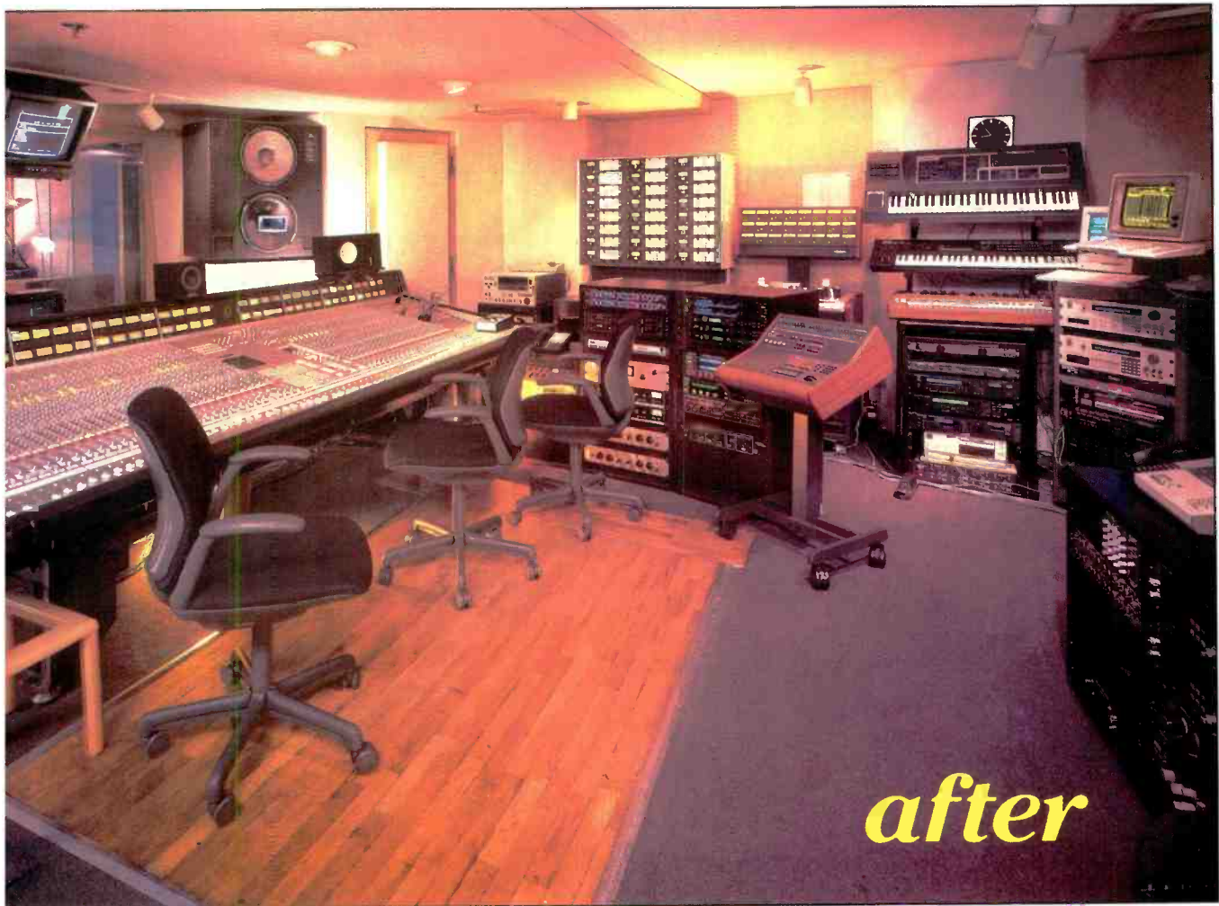
After: Note the acoustical shaping of 39th Street's front wall, including sound-rated laminated glass, new monitor soffits and isolated concrete mounts.
