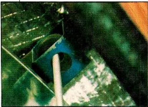
Photo 7. Duct isolator. Field inspections during construction are necessary to avoid improper construction and installation. If detected before the installation of finished materials (ceilings and wallboard, for example), conditions such as the misaligned ventilation duct hanger shown above can be corrected easily.
