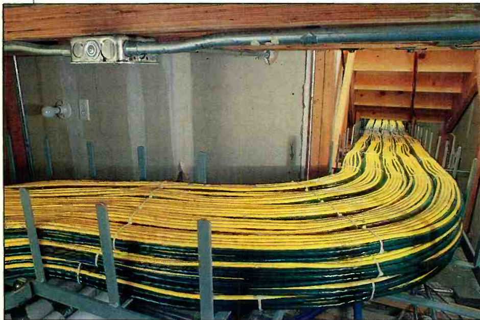
Photo 6. An example of the many wiring troughs.
