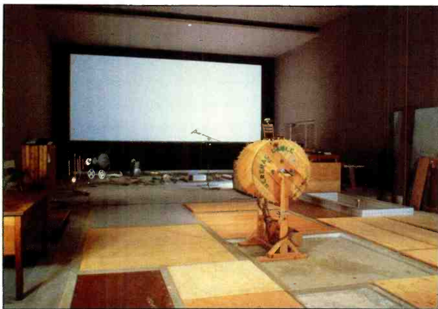
Photo 5. Foley stage. The design of the foley stage required the highest degree of sound-isolating construction to reach the background-noise criteria of NC-5, the single lowest background-noise criteria of the project.
