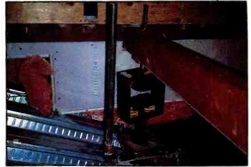
Photo 1. Ceiling isolator. The "room-within-a-room" design is applied to all recording stages in the building. The spring isolation hanger shown above is the resilient structural connection between the concrete scoring stage roof-deck above and the sound isolation ceiling below.
