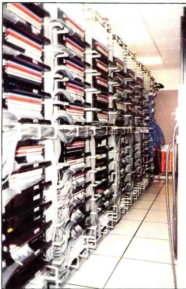
Photo 9. ADC cross-connect wall in a local machine room.
