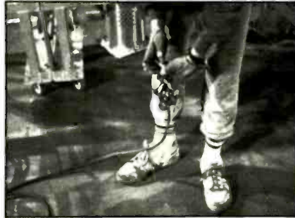
Figure 5. Rigger uses screw-pin anchor shackles to attach steel bridles to lifting line prior to hoisting.
