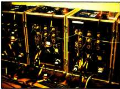
Figure 10. Power amplifier racks are loaded with Crest model 4000s.
