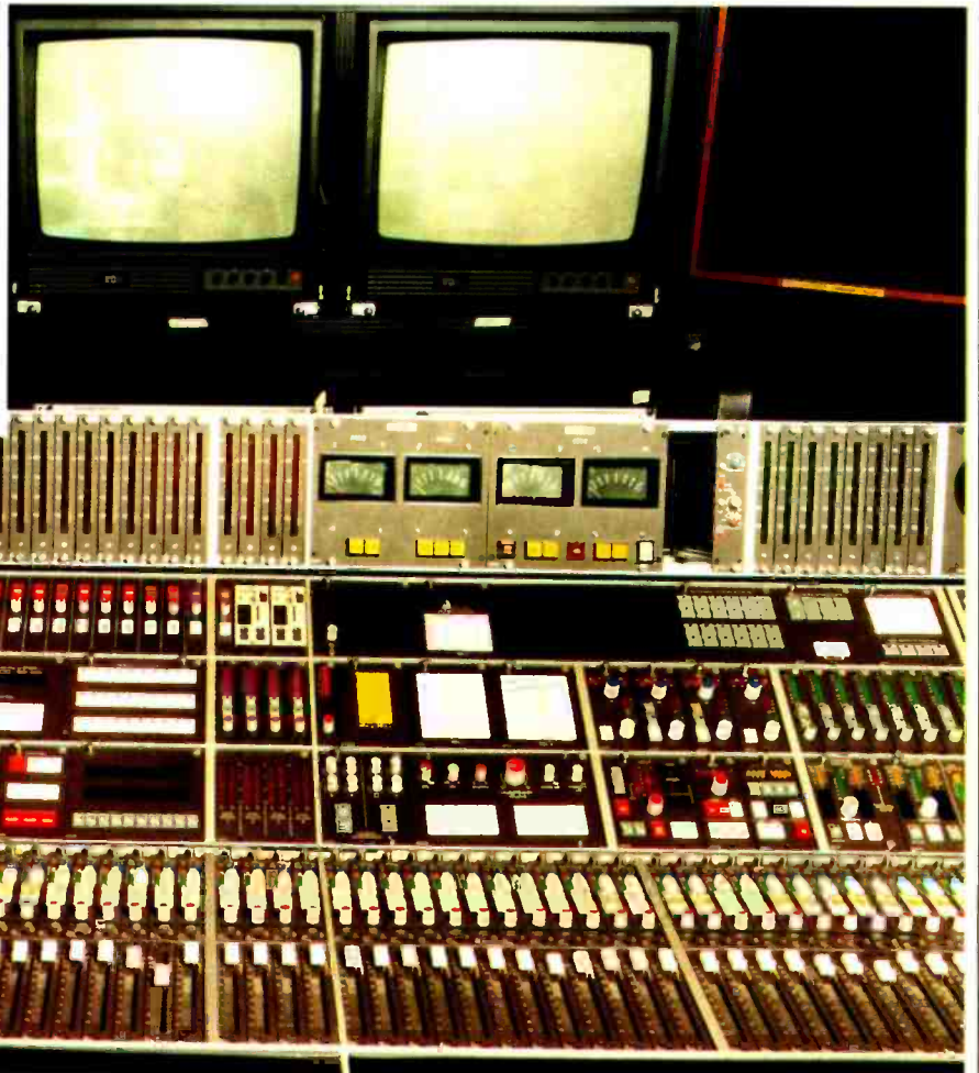
Section of an 112-channel assignable console for a BBC TV Master Sound Control Vehicle.
